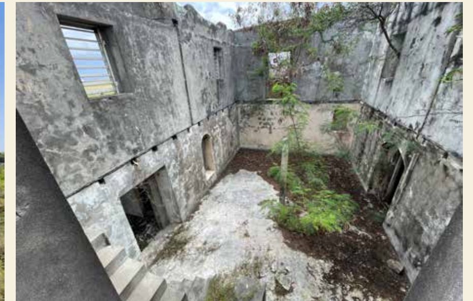
[Fig left] The nearly collapsed sugar mill of the Fair Play plantation.
