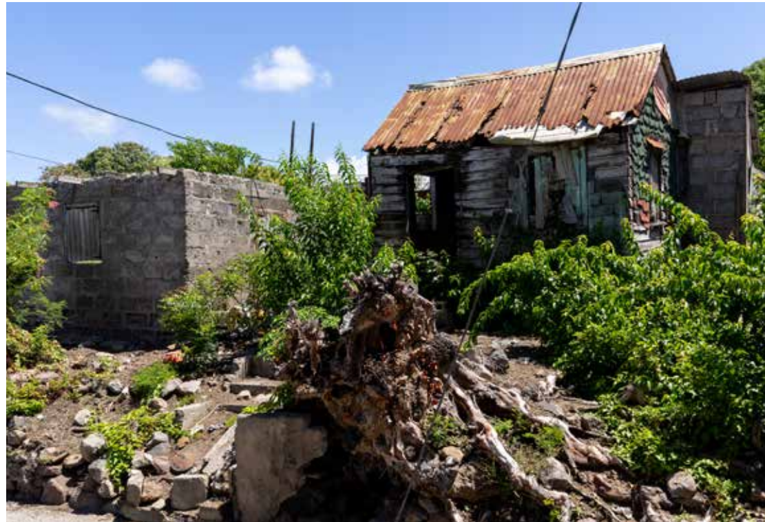
[Fig] Dilapidated house in Oranjestad.
