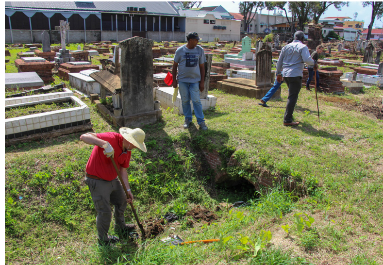
Work on the Nieuwe Oranjetuin in Paramaribo, Suriname – digging for information on the depth of the ditches in the cemetery (photo: René ten Dam)
